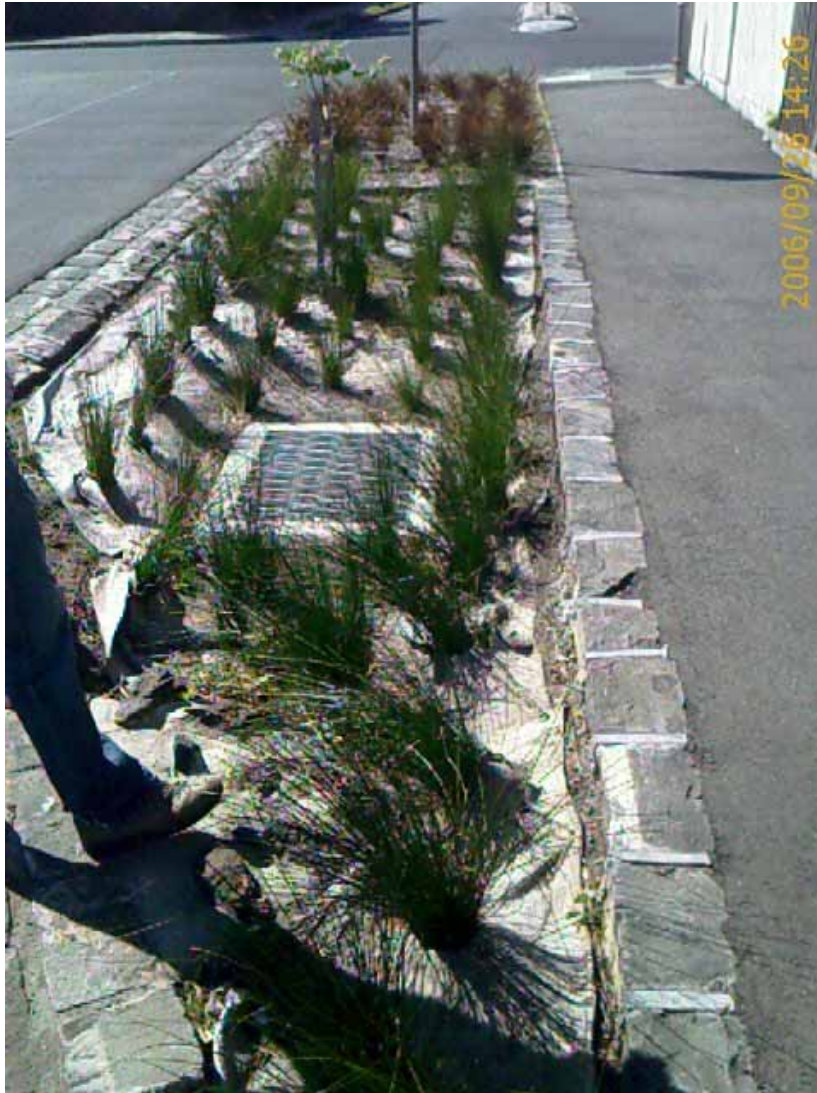
Figure 3-6 Rain garden with a blue stone edge, Hamilton Street, Brunswick West
