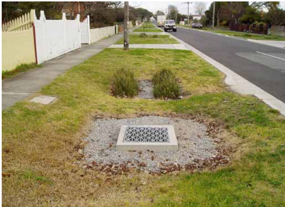
Figure 3-4 Grassed batters within a rain garden, Riviera Street, Mentone
