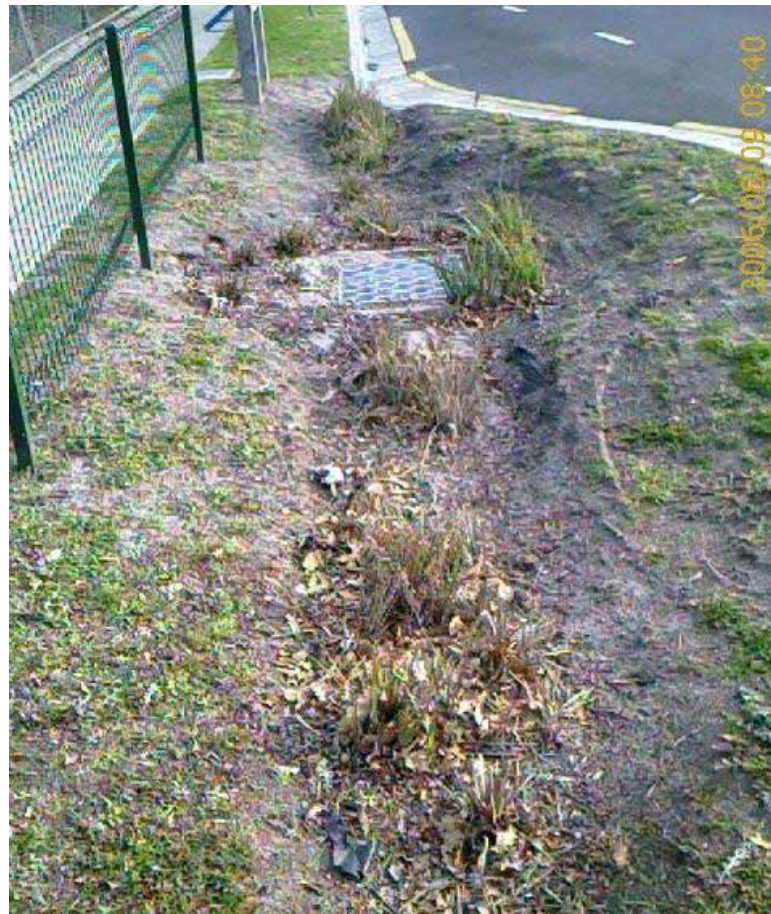
Figure 3-1 A rain garden in front of a school suffering damage from pedestrian traffic, Fowler Street, Bonbeach
