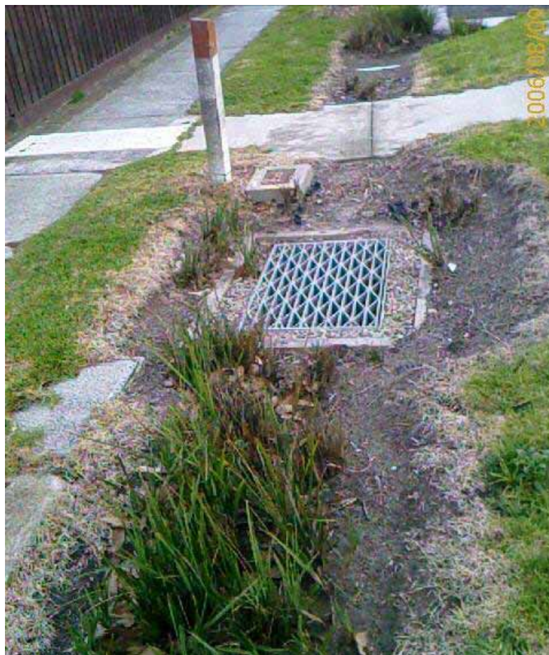
Figure 3-11 An example of the lack of edge strip and the effects of maintenance to keep grass clear of rain garden
